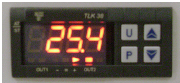
Figure 4-17 Stack Holder Power Supply Control Panel
