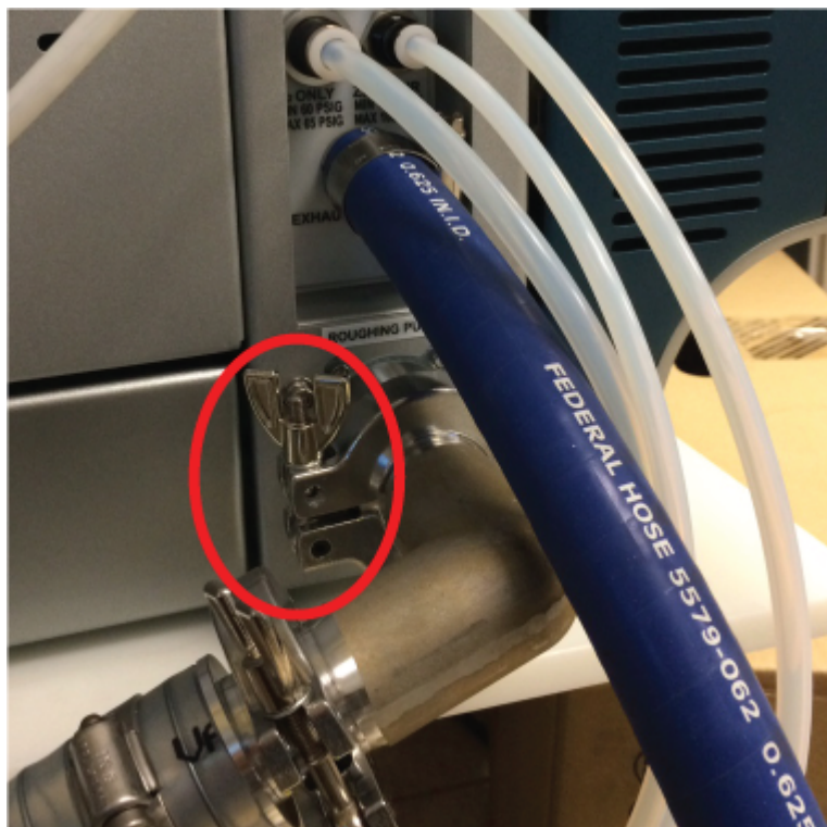
Illustration 5-15 : Collier correctement installé
